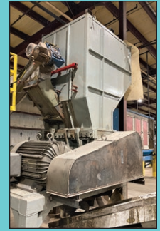
(2) 150 HP Cumberland Granulators
